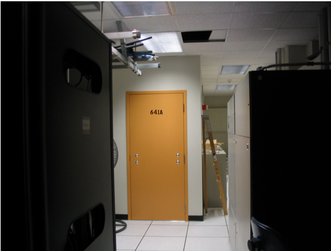
Entrances to the “secret room” at AT&T central office, 611 Folsom St., San Francisco
